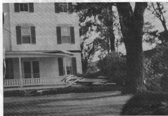
Memorial Weekend Storm Damage
