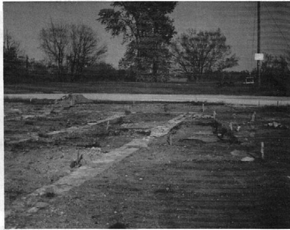
Photo shows Division Street in the background just past the bridge to be temporarily closed for boat launch construction. Foreground show foundation of old quarry store uncovered in site survey.
