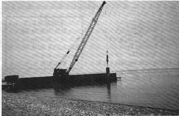
The work on the new dock for the Kelleys Island Ferry Boat Company continued even on New Years Eve. There is a chance service will start in the spring.
